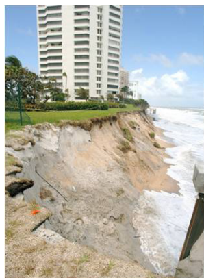
Hurricane-related beach erosion in South Florida
